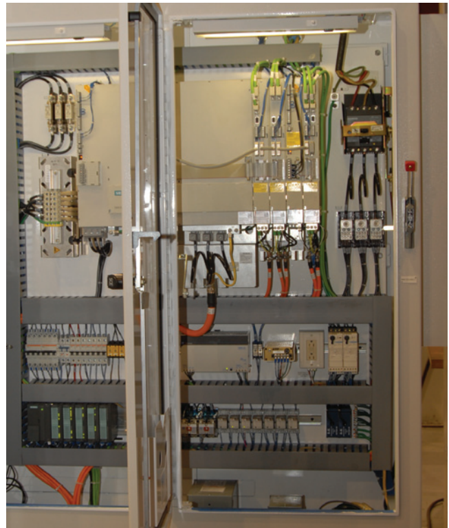
New electrical cabinet fitted with new built electrical panels
